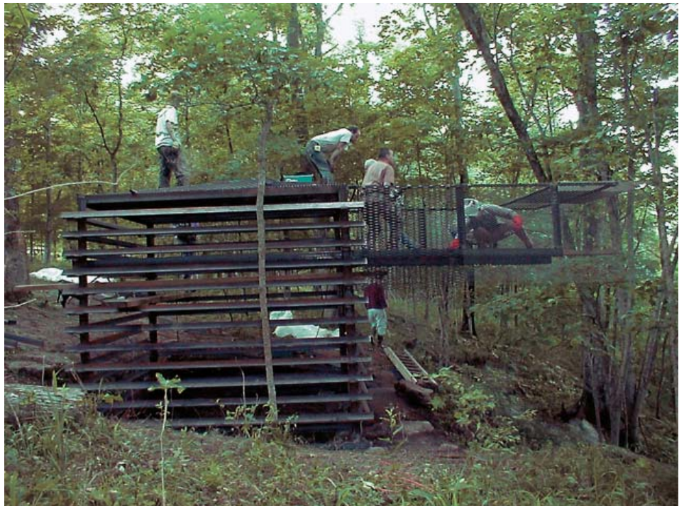
The construction of gates at the entrance of the Haile/Duds Cave in Jackson County, Tennessee, will protect habitat for rare cave species. Photo by Kristin Bobo
