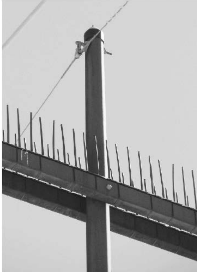
Figure 1. Raptor perch-deterrent devices (Zena, Inc., Odenville, AL) used on cross-arms and pole-tops of H-frame power-line support structures in southwest Wyoming, USA, in 2007.
